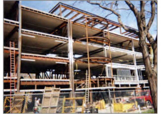
PHOTO COURTESY OF BRENDA BUTLER CRANSTON HALL BEING BUILT LARGER. ERIE WAS EXTREMELY BUSY THEN.
